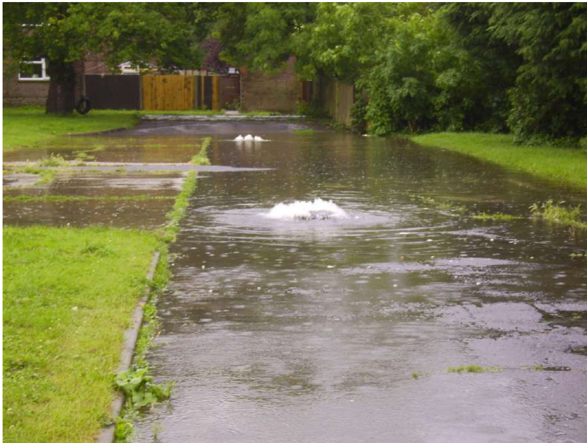
Figure 4.5 - Flooding from Public Manholes (June 2012)
