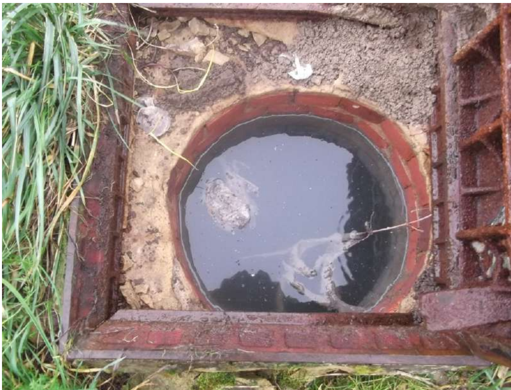
Figure 4.7 - Surcharged manhole (SU94036201) upstream of the Lidsey STW Feb 2014
